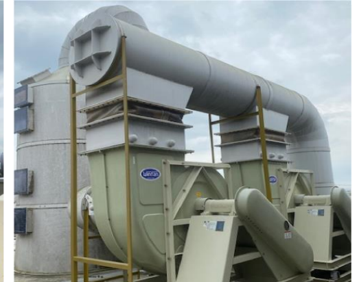
Dust collector tower
